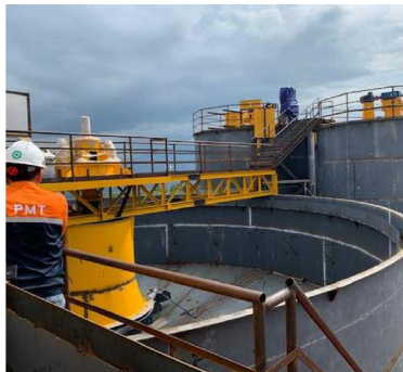
Thickener & Leach Tanks
